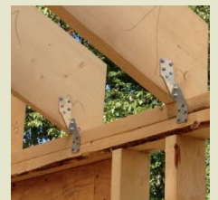
Hurricane clips on roof trusses
